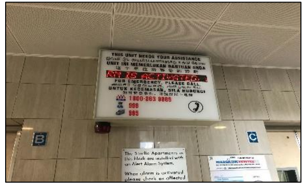
Alert alarm system at lift lobby
